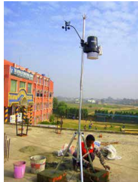
Automatic Weather Station installed on the top of the school building
