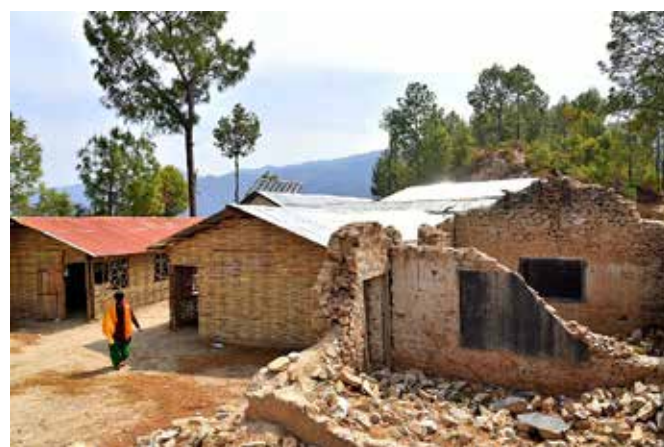
One year after Nepal Earthquake, this affected school has not been reconstructed yet. Lessons are being conducted in temporary learning centers (TLCs)
