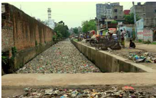
Open drainage full of garbage
